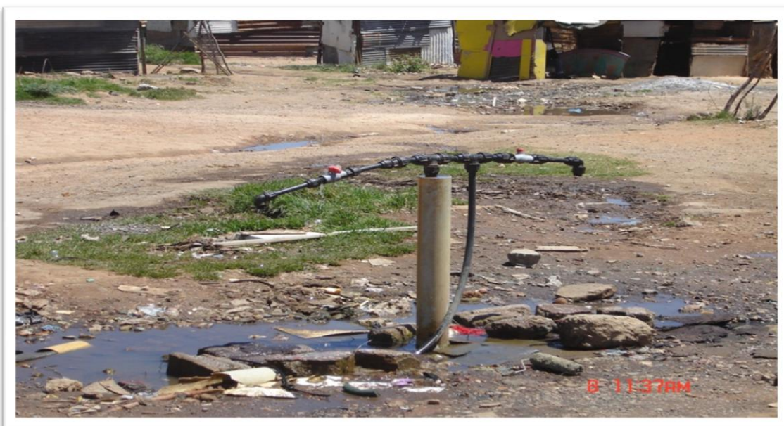
Photo 2: Communal tap in Case study 2 informal settlement (taken by the researcher)
